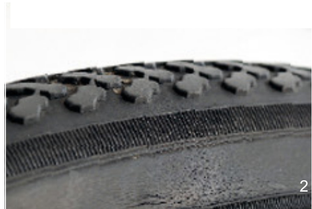
Figure 163: Examples of fatigue cracks (1) and ageing cracks (2)
